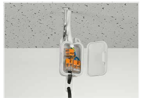
Pendant light connection in suspended ceilings
