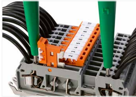
Testing with voltage tester.
