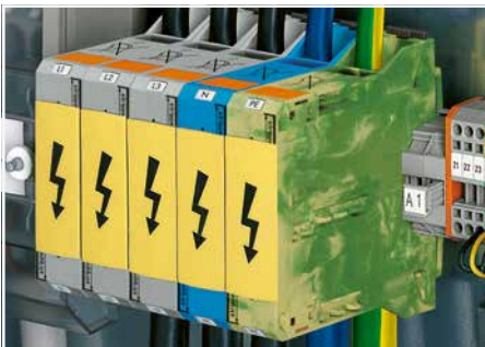
Protective warning marker may indicate: Notice: Power is still on even after switching off the main switch!
